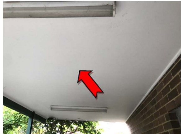
Photo 4. Exterior, rear verandah, awning – assumed asbestos-containing fibre cement sheeting.
