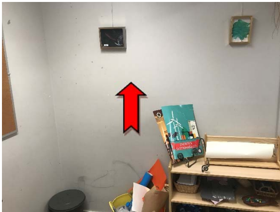
Photo 1. Interior, ground level, north eastern playroom, northern wall panels – asbestos-containing fibre cement sheeting.
