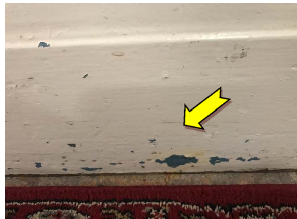
Photo 6. Interior, throughout, skirting board – suspected lead-containing cream upper paint system.
