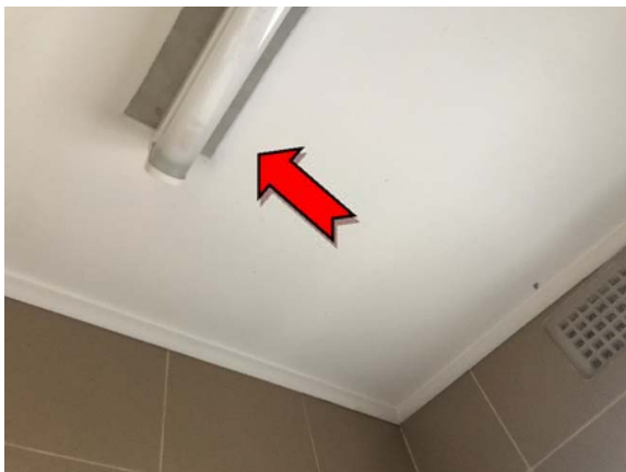
Photo 5. Interior, ground level, nappy change room, ceiling – assumed asbestos-containing fibre cement sheeting.
